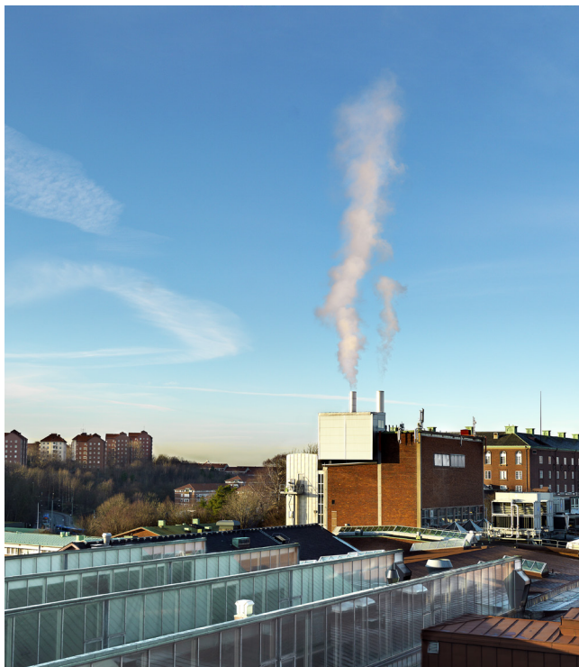
Chalmers 12MW boiler
