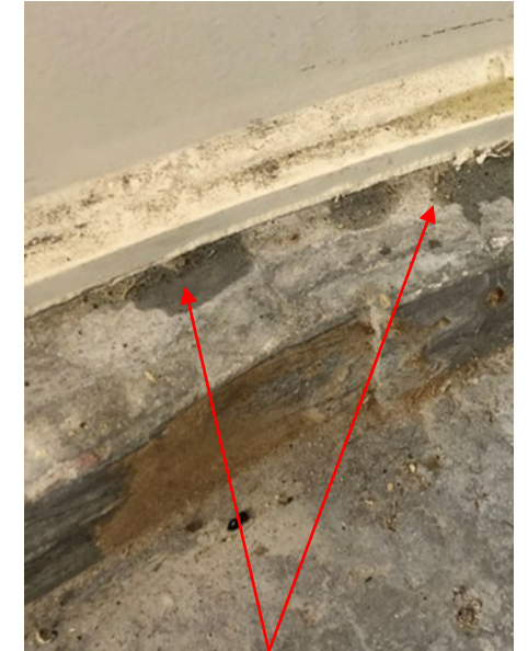
Inward leakage of water
