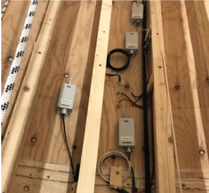
Positions of RH and T sensors and electrodes for moisture content measurement
