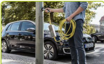
Simple Socket & Smart Cable - Lamp Column Charging Point
